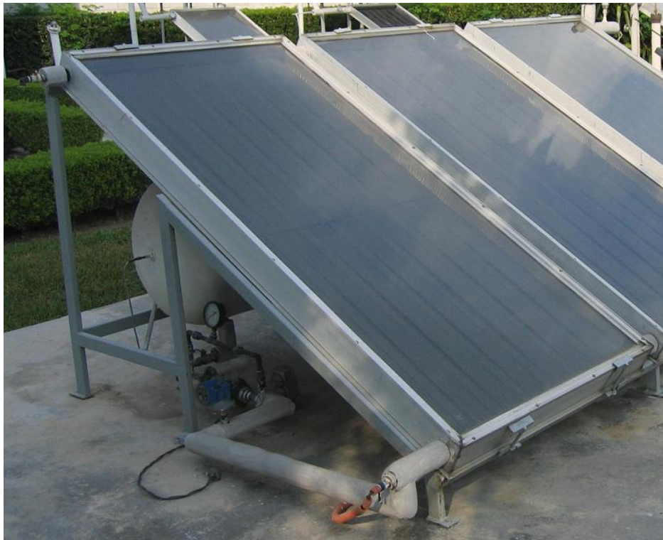
Fig 3. Flat plate solar collectors at “Casa Solar” from Tecnológico de Monterrey
